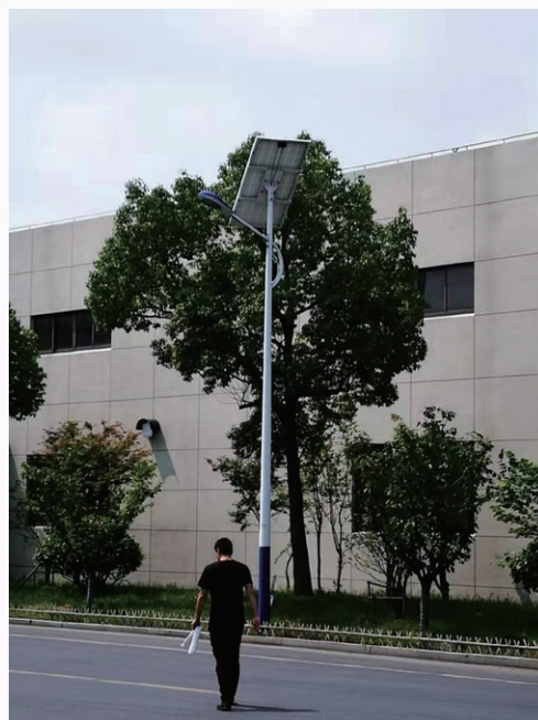
Outdoor solar street lights 室外太陽能路燈
