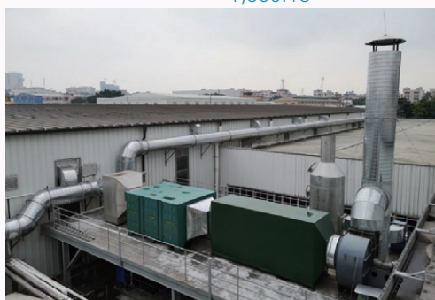
VOCs and ammonia collection and treatment system VOCs及氨氣收集處理系統
